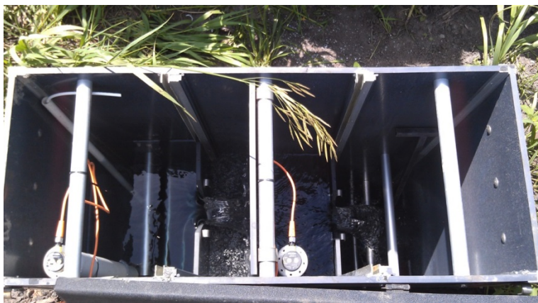
A typical control structure, equipped with water level sensors, v-notch weirs, and splash guard between chambers
